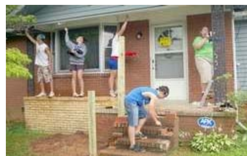
Carol Hoglen/The Dispatch Group WorkCamps members Tony Chretien (from left), Kirsten Flennig, Emily Trudeau, Trey Reuther and Kimberly Homan paint and lay bricks on the front porch of Nellie Holt's house on Thurgood Avenue. The Lexington Housing Community Development Corp. is hosting approximately 400 high school students during this year's Group WorkCamps session.
